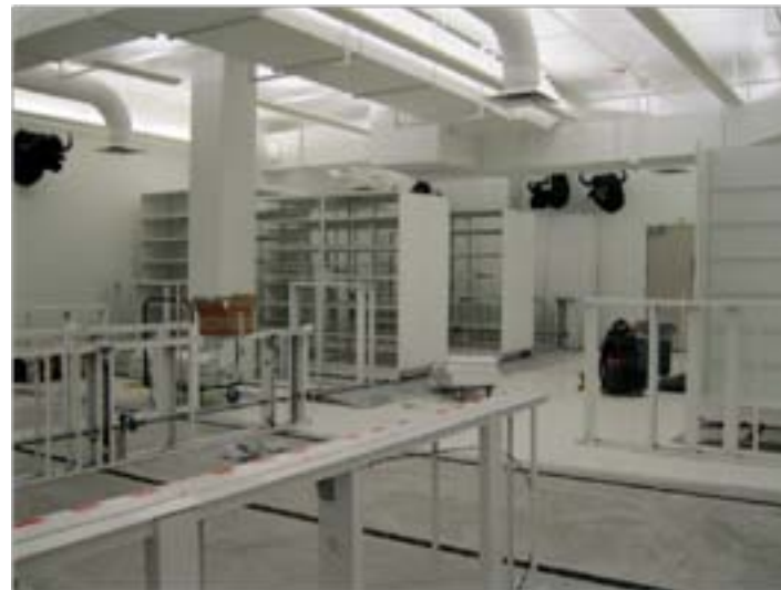
Figure 2. Construction and installation of three different compactor mobile storage sections (left, open shelving; right, closed shelving; front, cabinets).
